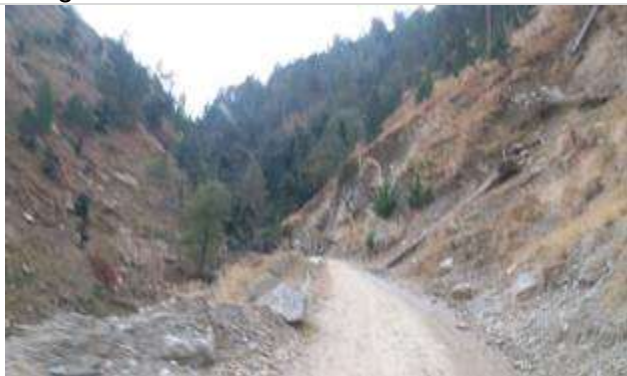
Sliding area Ch 2+600
