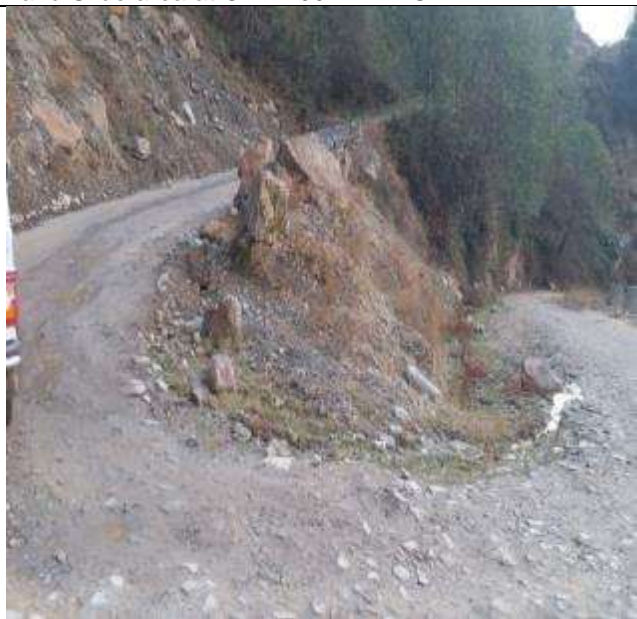
Sharp Turning and Poor Gradient at Ch 6.100 Km
