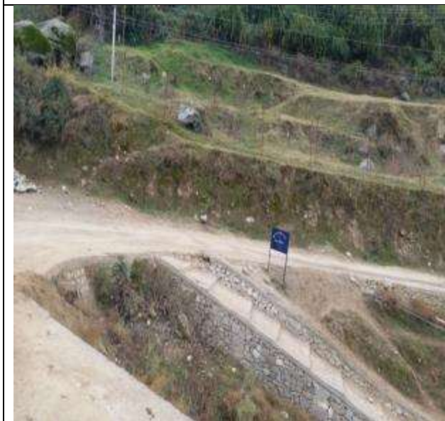
Poor road condition at Ch 3.800 Km
