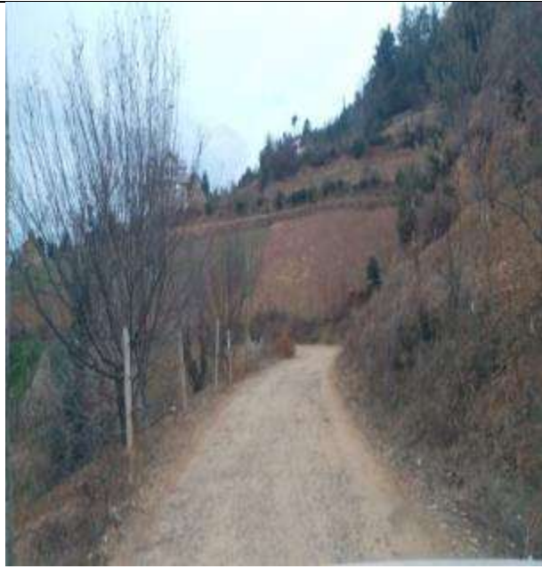
Road condition at Ch10.000 Km
