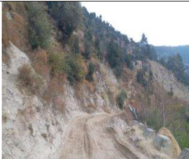
Land Slide area at Ch 2.400 Km LHS
