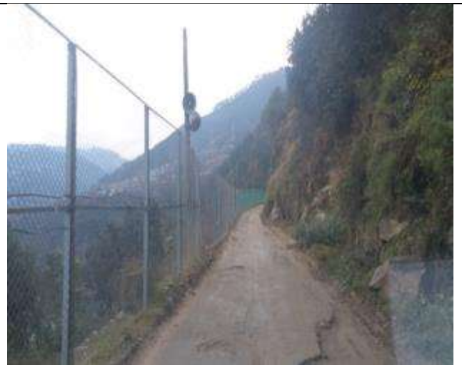
Poor Road Condition at Ch 1.000 km
