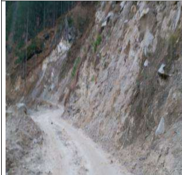
Land slide area at Ch 6.000 Km
