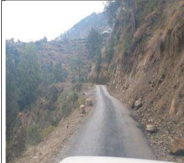
Land slide area at Chainage 1.800 Km
