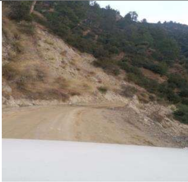
Land Slide area at Ch 1.100 Km
