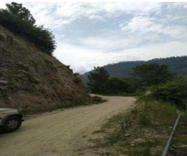
Land Slide Area at Ch 0.0150 km
